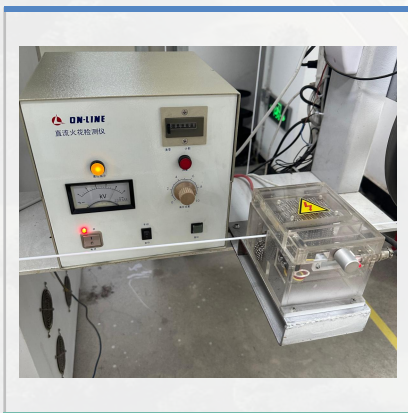
Withstand Voltage Monitoring
